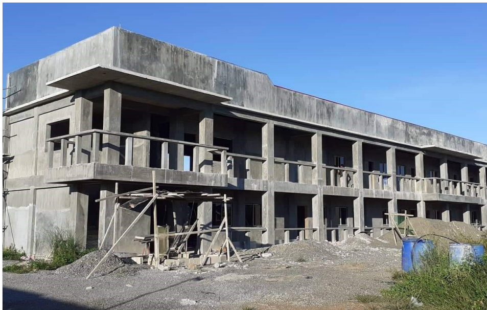
The Engineering & IT Building with project cost, PhP 15,673,633.92, at IFSU Potia Campus was completed in February 2019.
