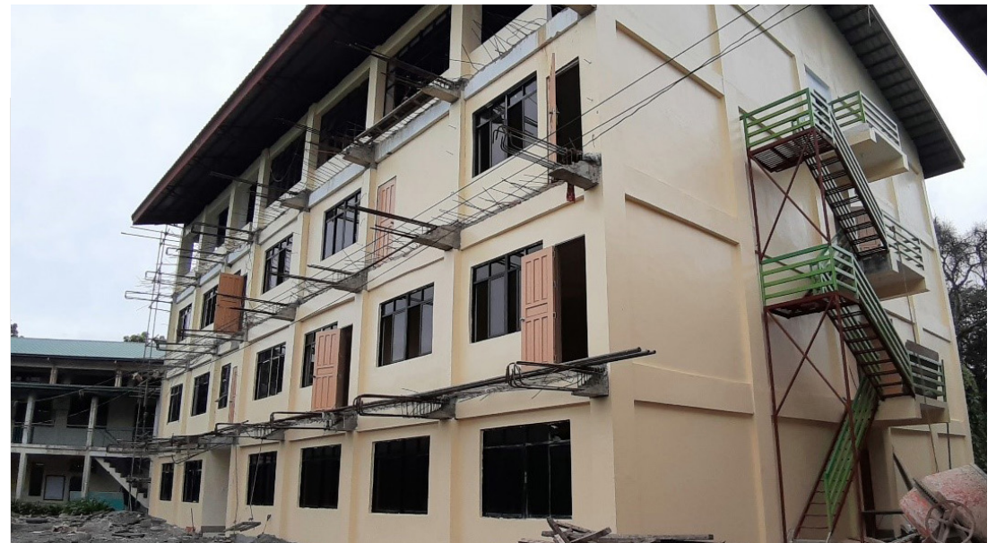
The Hostel Cum BHRM Laboratory Building (Phase 2) with project cost, PhP12,848,738.32, at IFSU-Lagawe Campus was completed in June 2019.
